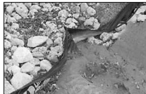
A section of silt fence is partially buried by mobile sediment at an active Texas construction site. Regulatory agencies and private interests are increasing their demands for more effective storm water controls.
